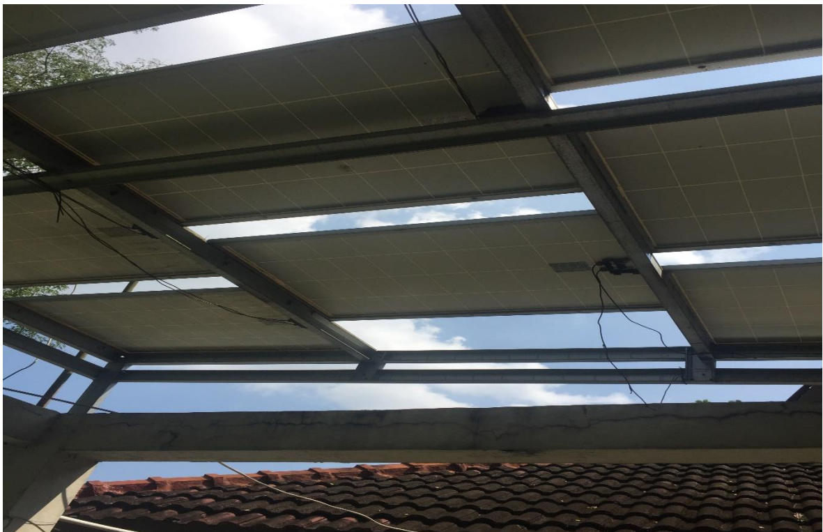
Gambar Lampiran 1. 2 2 Sollar Cell / Panel surya
